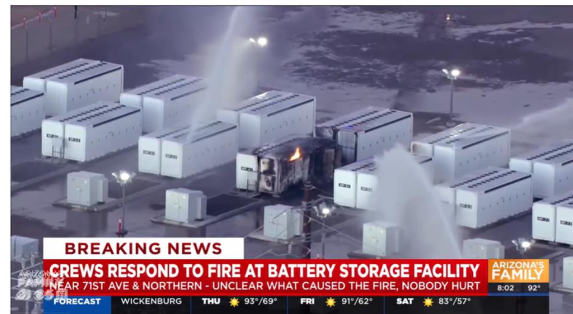
The Salt River Project, known as SRP, is aware of the fire at its 25-megawatt battery system at its Bolster substation. Stephanie Duprey reports.
